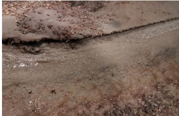
Figure 21: Photograph of the left bank of the flume after the running of the sequence of floods
