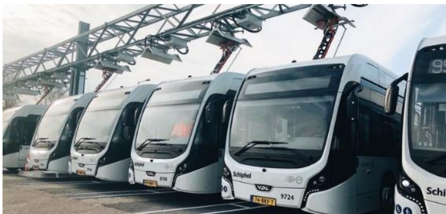
Figure 2 Pantographs installed in the depot (Source: Siemens, https://new.siemens.com/global/en/company/stories/home.html )
