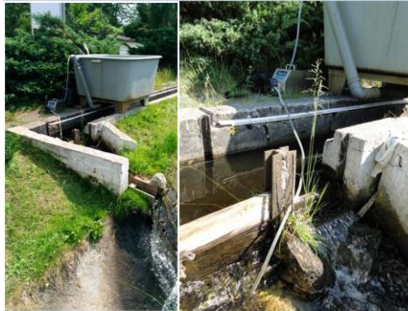
Figure 10 Pump and mixing water system, source: Florian MIROLO
