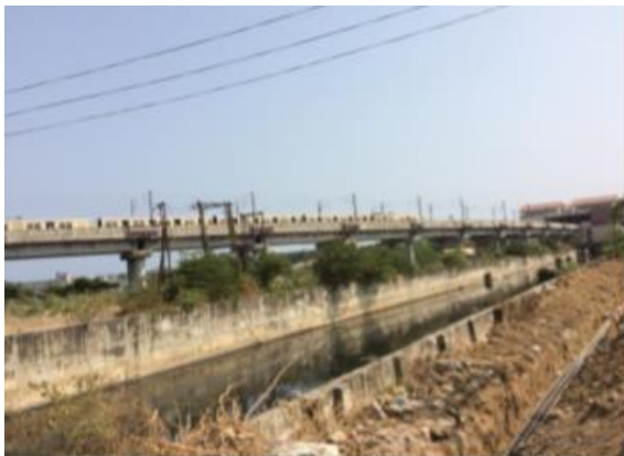
Figure 18 Culvert with inadequate capacity
