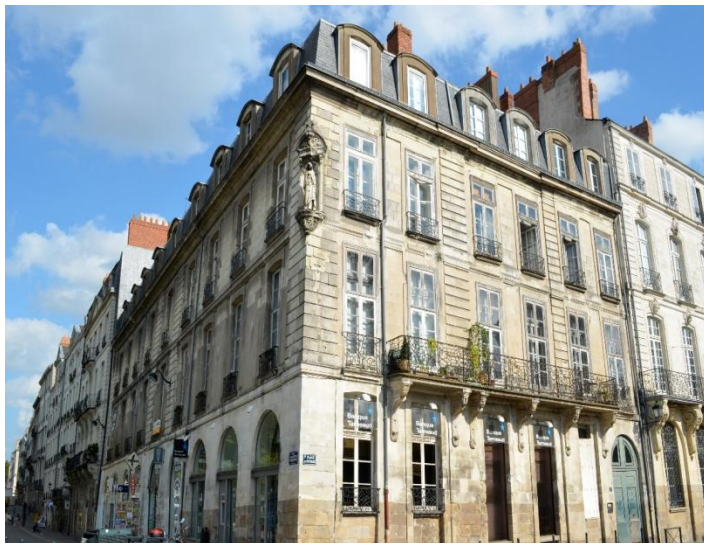
Fig 1.22: House in dilapidated condition
