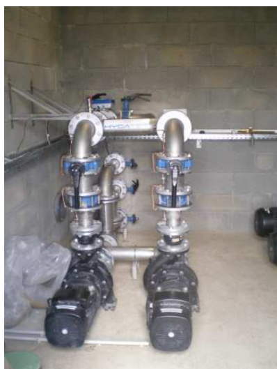
Figure 50: Pompes du local technique
